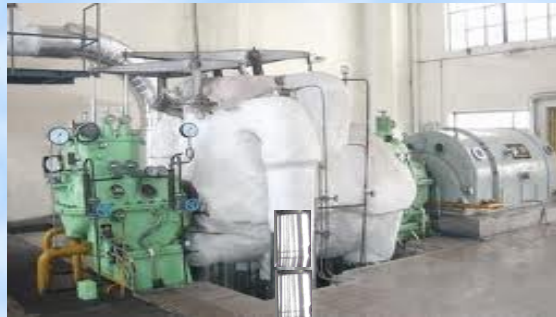
Direct Condensing Low Pressure Turbine Generator
